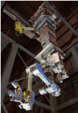
Many Overhead Telescopic Manipulator Systems are in service at all the DOE nuclear facilities doing a wide variety of remote operations, e.g., decontamination, maintenance, and size reduction activities in very tight closed spaces found in hot cells and glove boxes.
